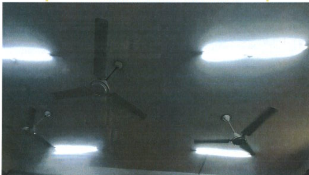
Site photograph 1 Classroom conventional fan
