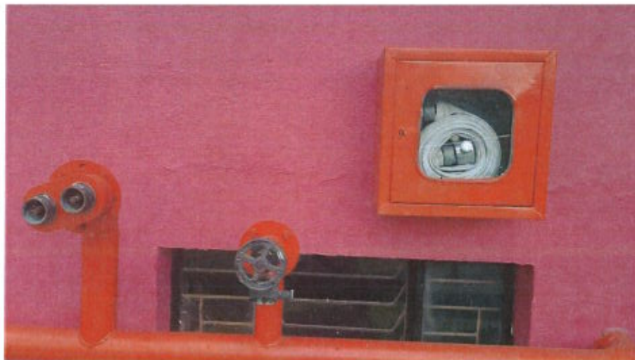
Site photograph 4 Fire Safety Pipeline and Hose
