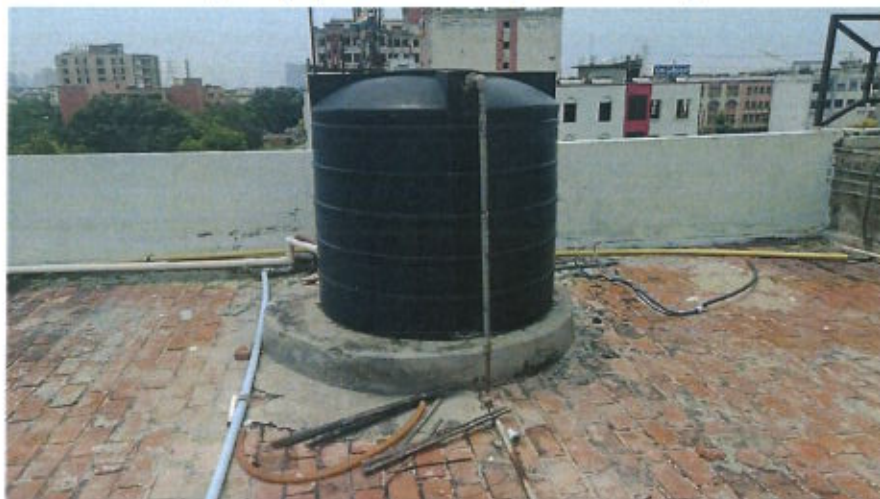
Site photograph 2 Water Storage Tank in Campus
